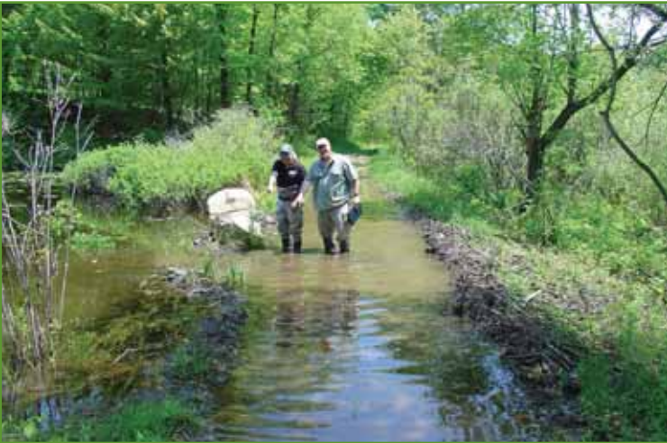
Figure 23. Flow to south from Edwin Butcher Wildlife Pond to East Mud Lake, NY (Note: beaver-blocked culvert at south end of Edwin Butcher Wildlife Pond). Photo from USACE.
