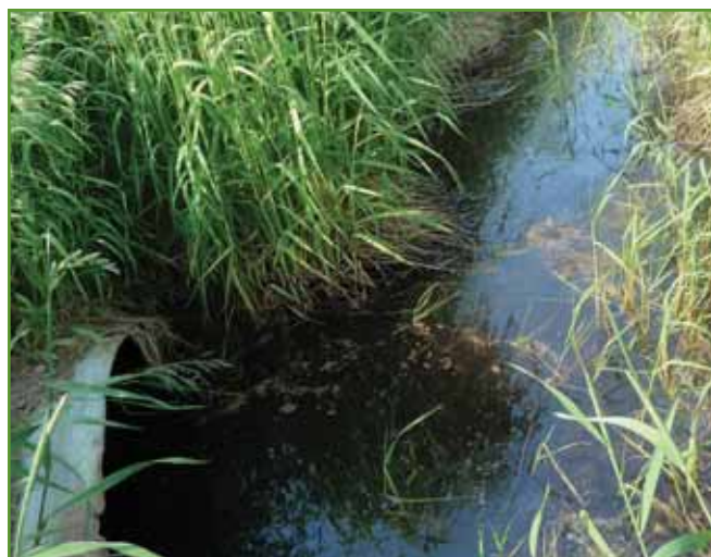
Figure 62. Existing four foot culvert under County Road M. Photo taken on wetland side (west) of the roadway. Any flow across the basin divide is constrained through this culvert. Photo from USACE.
