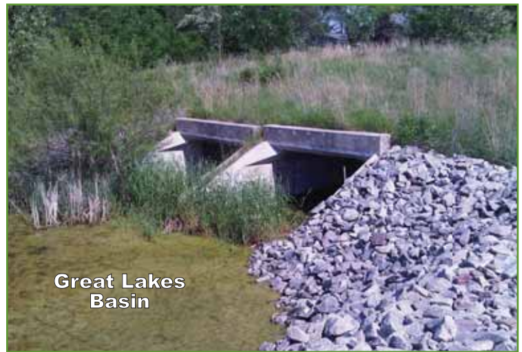
Figure 56. Portage Flood Risk Management Project Un-gated Interbasin Flow Structure. Photo from USACE.
