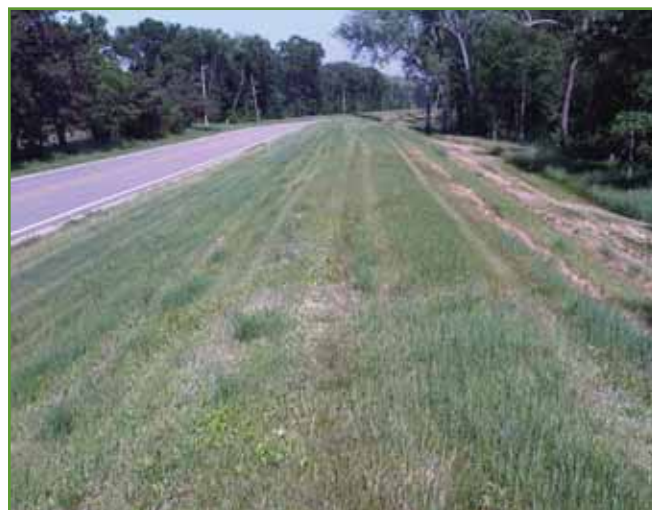
Figure 59. Lewiston Levee along County Road O which forms basin divide at Portage Upstream Locations. Photo from USACE.
