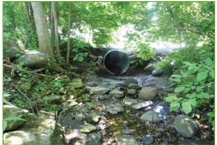
Figure 53. North end of urban storm drain near Ann Avenue (looking south). Photo from USACE.
