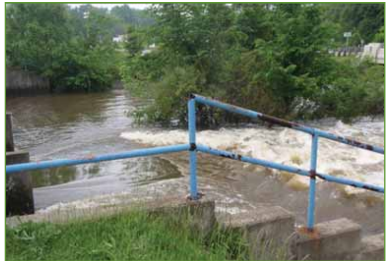
Figure 38. Outlet from Long Lake Flood Gates during May 27, 2011 site visit, forming headwaters of the Tuscarawas River. Photo by USACE.
