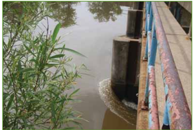
Figure 37. Intake to Long Lake Flood Gates during May 27, 2011 site visit. Photo by USACE.
