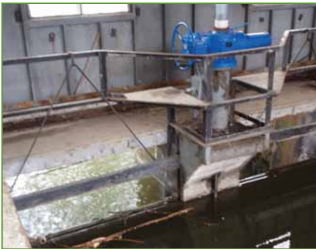
Figure 40. Lock 1 North Control Weir. Photo from USACE.
