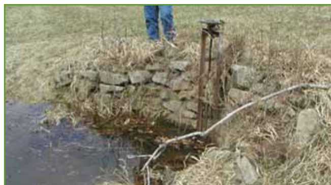
Figure 61. Culvert Under Lewiston Levee at Potential Connection Number 1 Shown on Figure 54. Photo from USACE.
