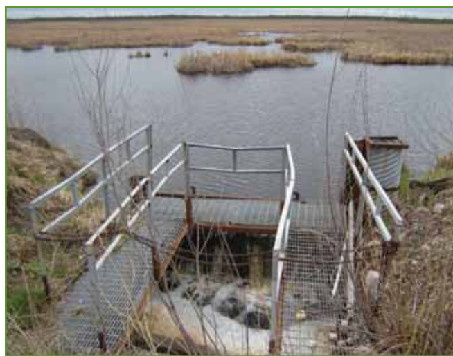
Figure 18. View of drop structure at US Route 2, looking southwest. Photo from USACE.
