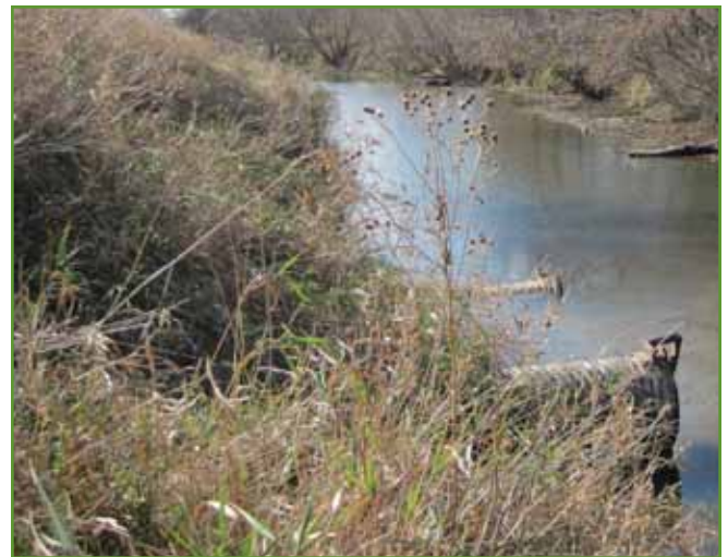
Figure 9. 12-inch pipes through Graham McCulloch Ditch left bank berm. Photo from USACE.
