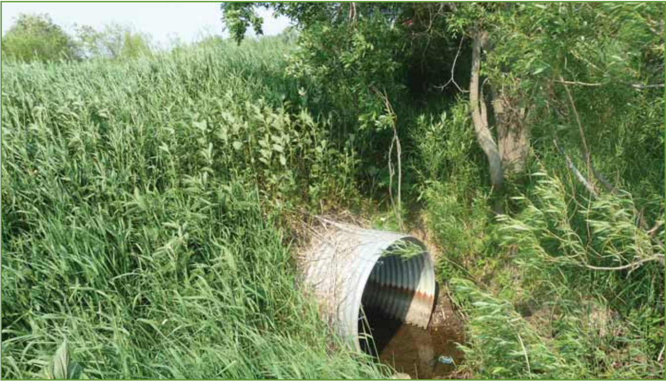
Figure 12. Photo at Davis Road, looking at the three-foot CMP on the south face of the culvert. Photo from USACE in 2011.
