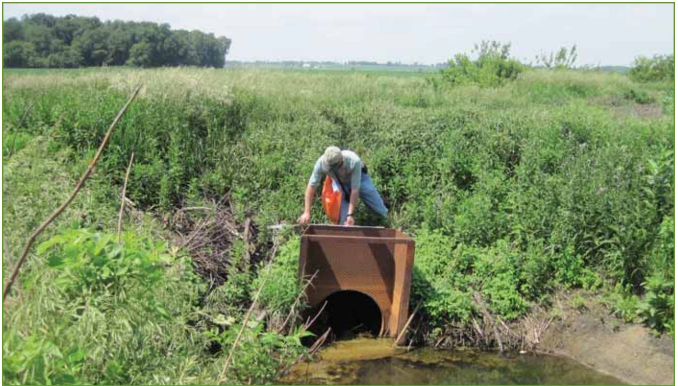
Figure 10. View looking southwest from east bank of West Fork Parker Ditch showing metal headwall and 27-inch (69cm) CMP culvert that extends approximately 40-feet (12 m) and connects with Parker-Cobb Ditch. Photo by USACE.
