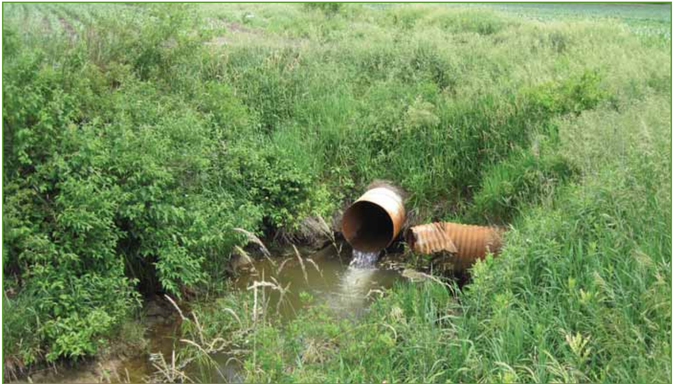
Figure 11: Water flowing into Parker-Cobb Ditch through 27-inch (69 cm) CMP from West Fork Parker Ditch. Photo by USACE.
