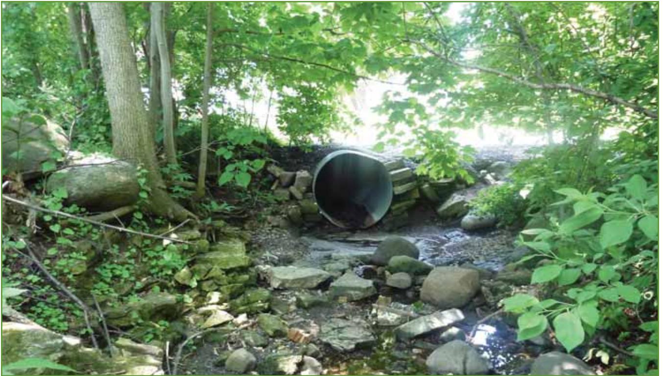
Figure 22. North end of urban storm drain near Ann Avenue (looking south). Photo from USACE, June 2011.
