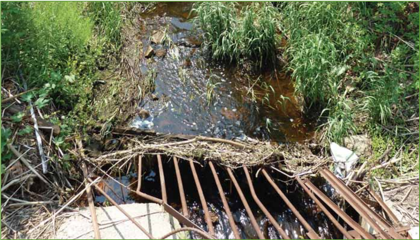
Figure 25. South end of urban storm drain near Menomonee Avenue, looking towards Tamarack Swamp. Photo from USACE, June 2011.
