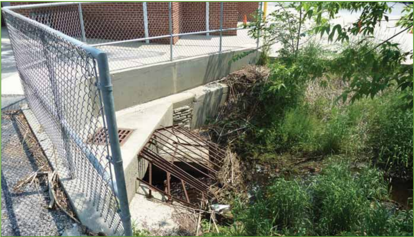
Figure 24. South end of urban storm drain near Menomonee Avenue, looking at culvert entrance. Photo from USACE, June 2011.
