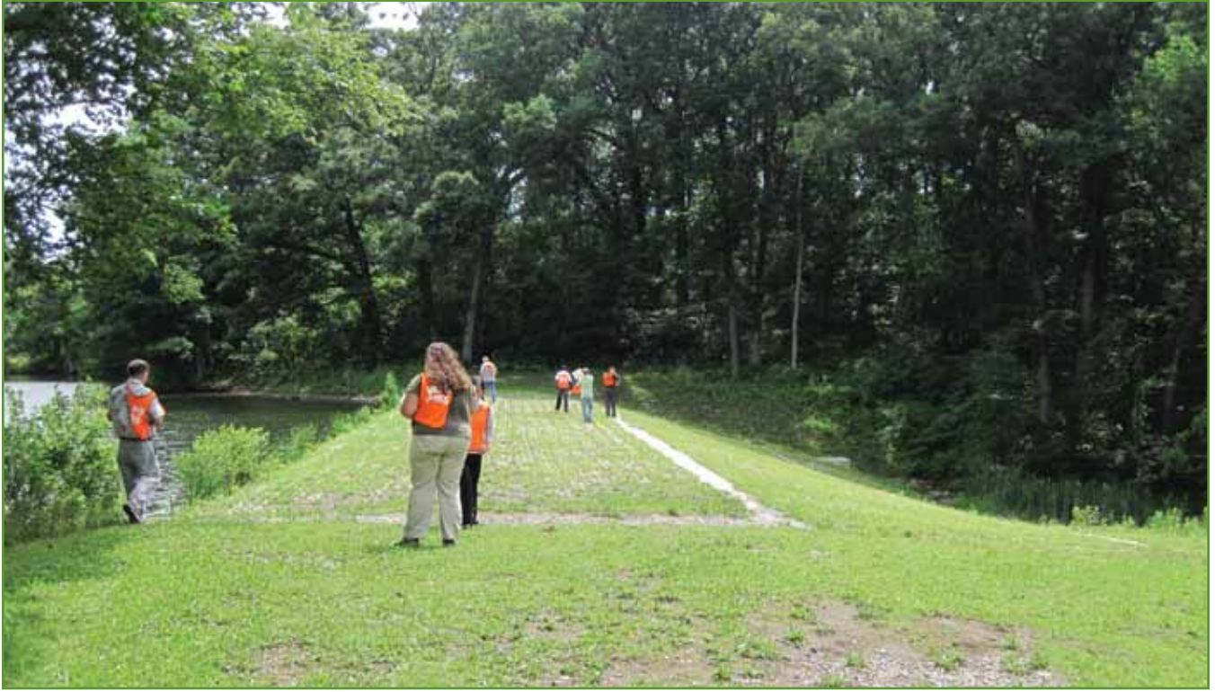
Figure 10. Proffitts Dam on Loomis Lake, looking southwest. Photo taken June 20, 2011 by USACE.
