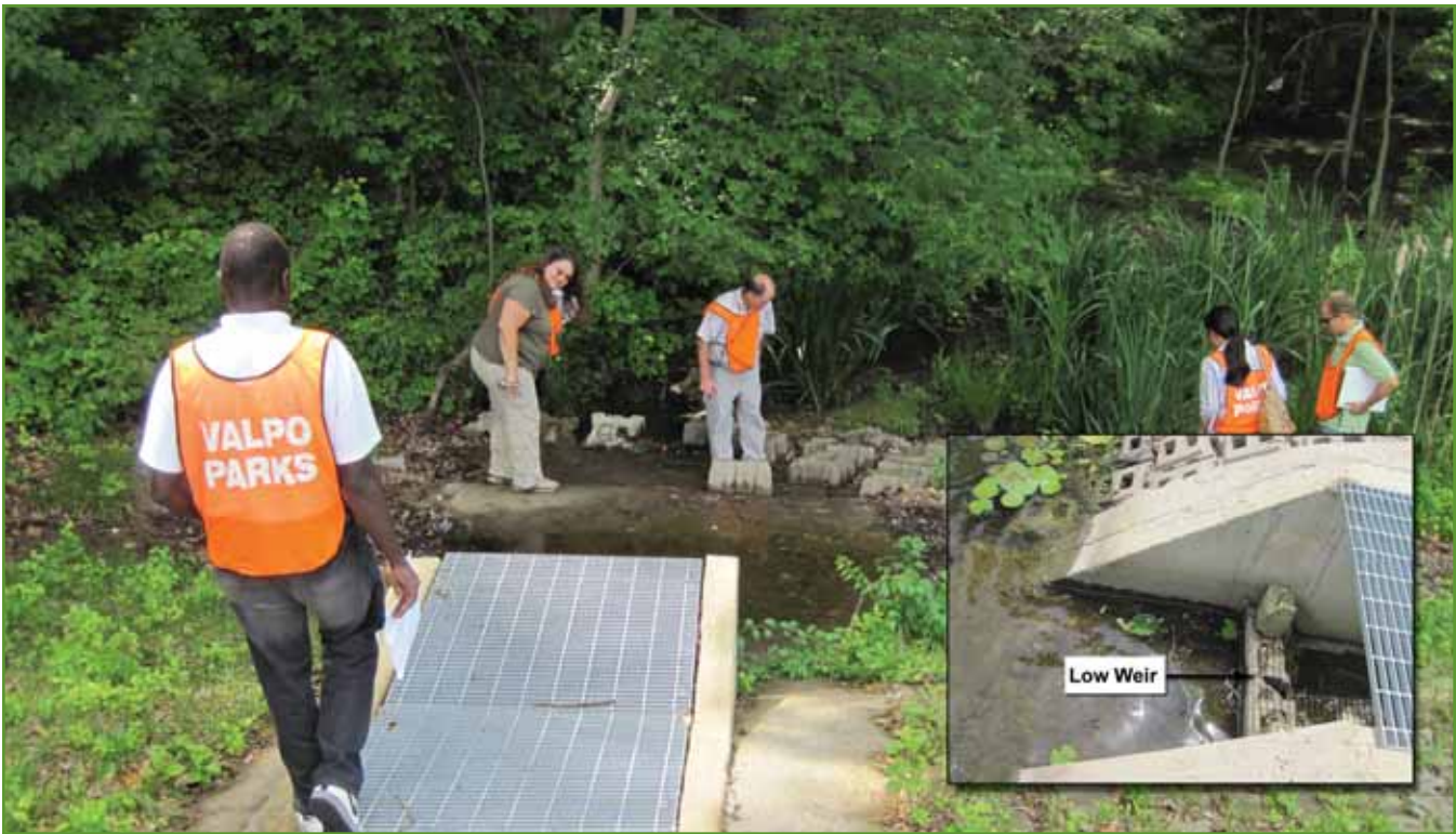
Figure 15. Loomis Lake 3 foot (0.9 m) square (approx.) concrete channel auxiliary spillway to Damon Run, looking downstream; (Inset) Entrance to concrete channel of this auxiliary spillway at Loomis Lake. Photos by USACE
