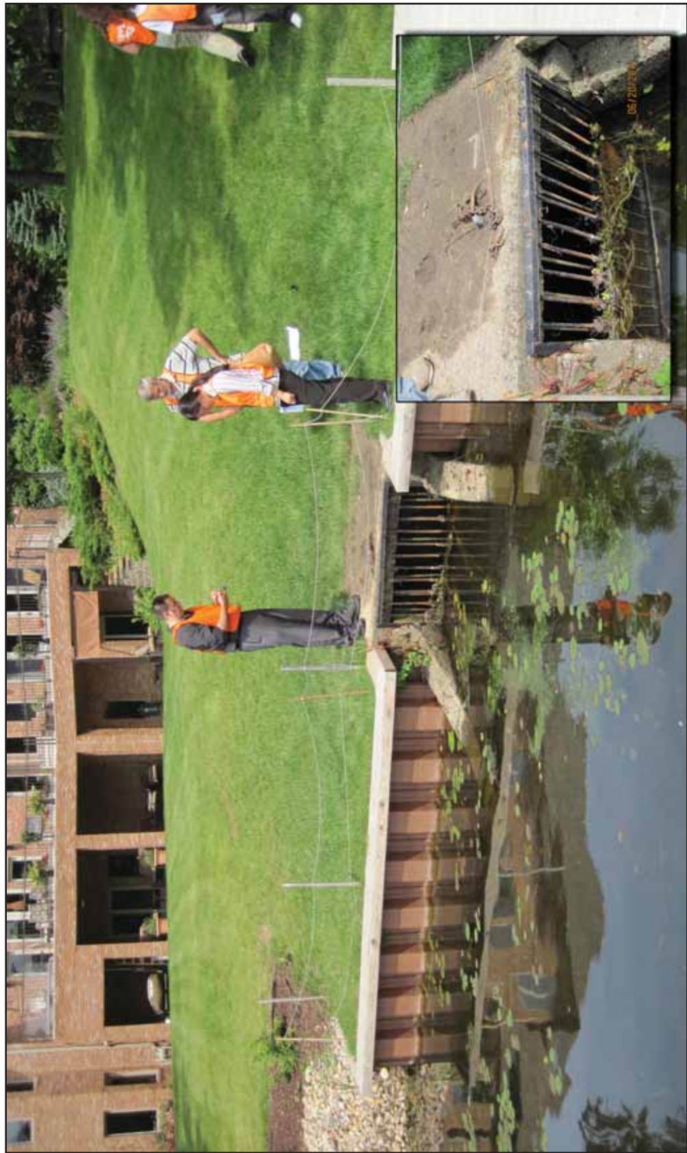
Figure 14. Loomis Lake grated drop box inlet structure for culvert to Flint Lake. This is the inlet to the 900-foot (274m) long underground culvert, facing east. Photo by USACE.
