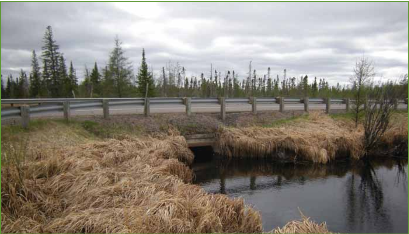
Figure 8. Culvert under US Route 2, southeast of intersection with MN-200. Photo by USACE.
