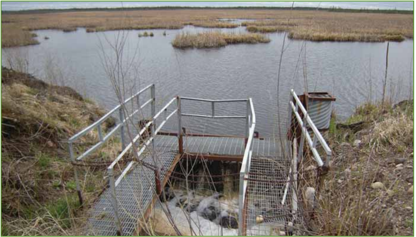
Figure 9. View of drop structure at US Route 2, looking southwest. Flow is to the Mississippi River Basin toward the bottom of the picture. Photo by USACE.
