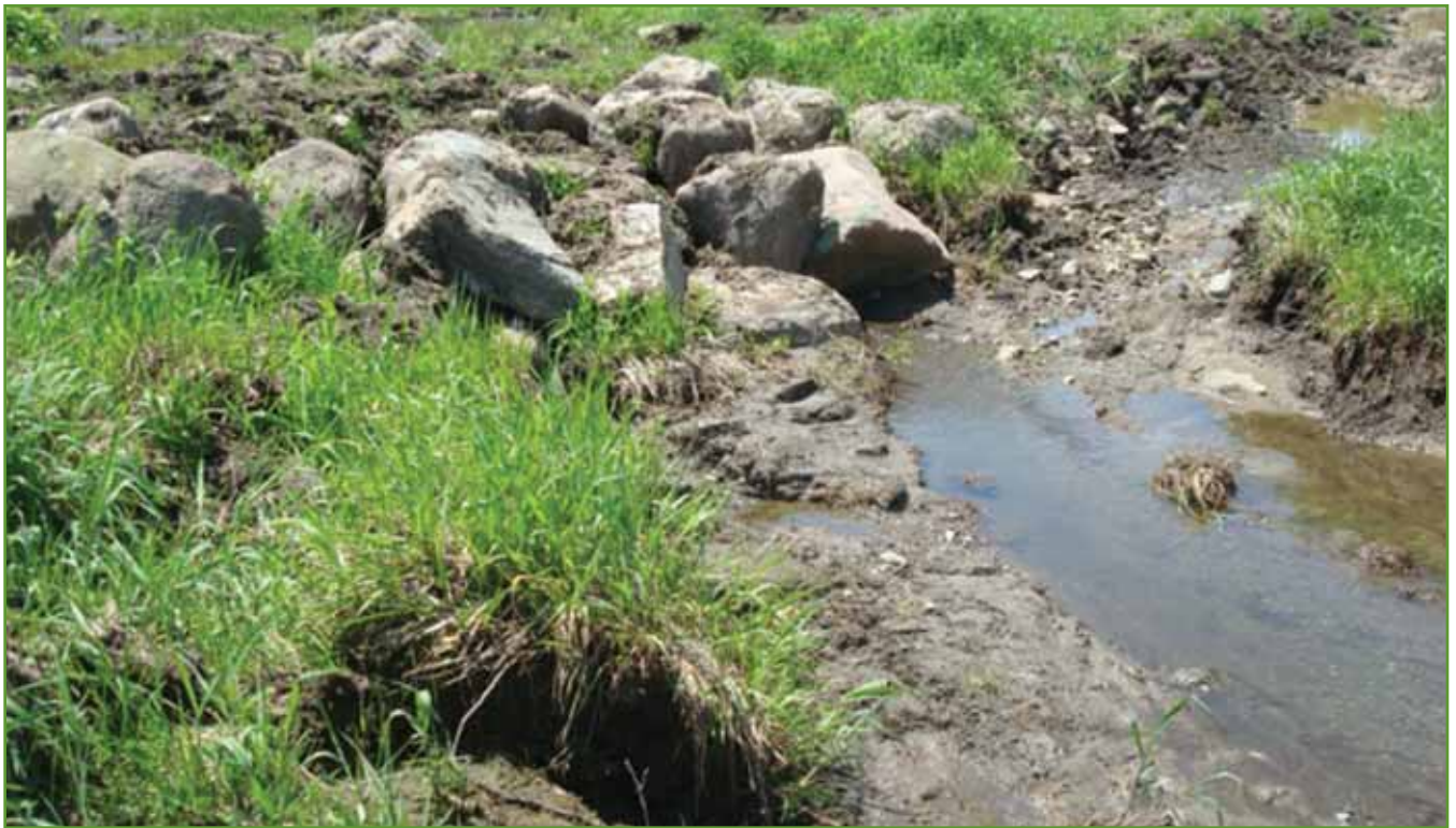
Figure 12. Farm road bridge in tributary to Silver Creek, north of the Edwin Butcher Wildlife Pond. Photo by USACE. Reference also Figure 13.
