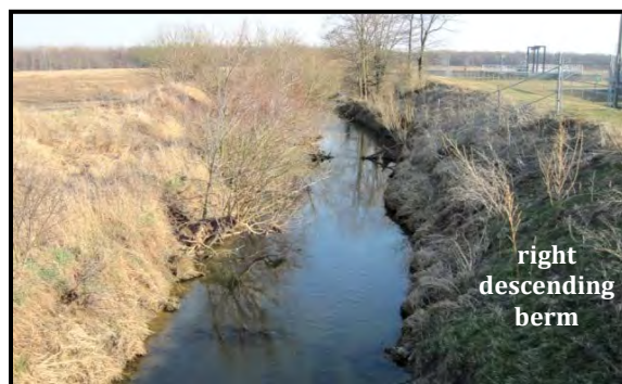
Photo 3.5: Graham-McCulloch right descending berm as seen from the water treatment plant access road, 14-Mar-12.
