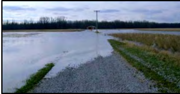
Photo 2.4: Flooding across the entrance road, 28-Apr-11
